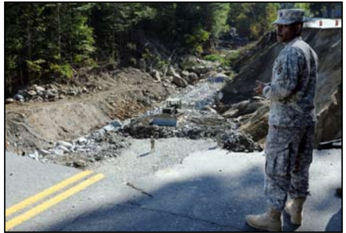
The Ohio National Guard helped fix a 65-foot-deep highway washout that followed Tropical Storm Irene in Vermont. Ohio has been supporting the Vermont National Guard’s Joint Task Force Green Mountain Spirit under a state Emergency Management Assistance Compact. SSG Jim Greenhill / NGB
